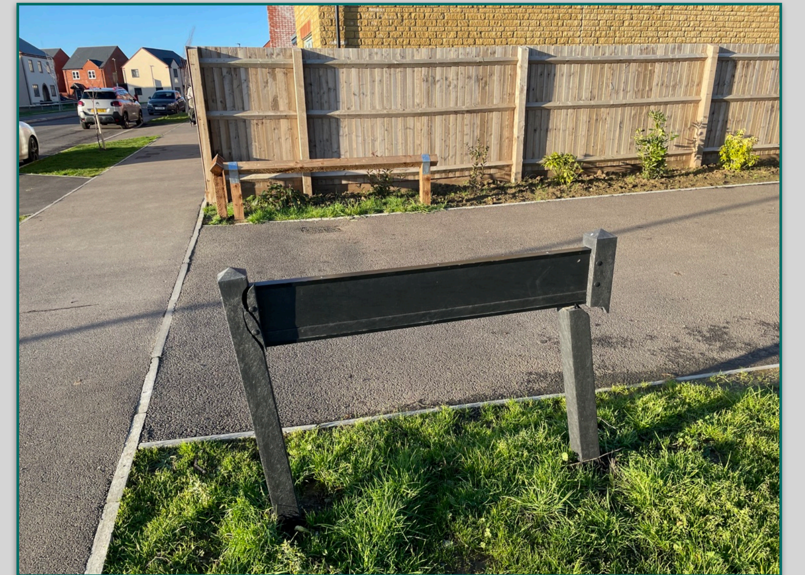
Broken Street Sign
